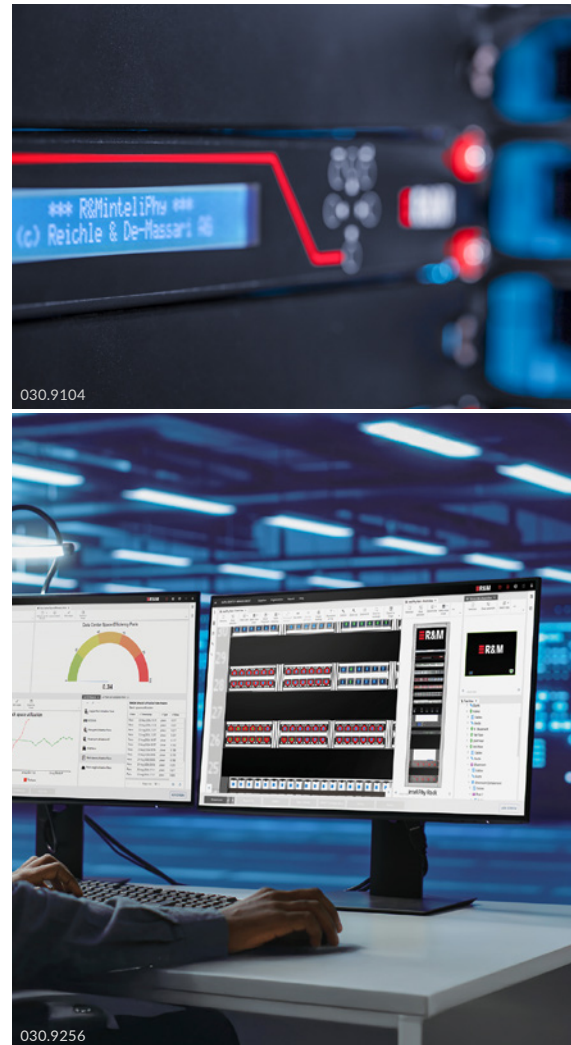
inteliPhy is increasingly becoming a digital architect for data centers.
