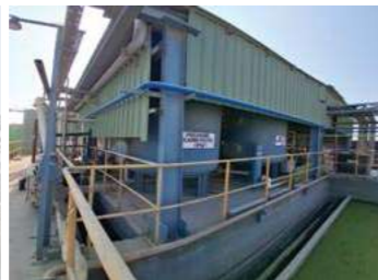
Sand Filter and Carbon Filter
