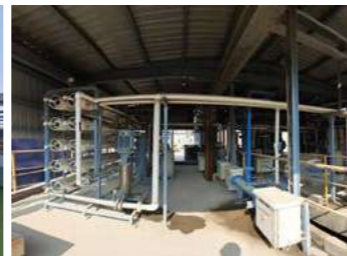
Ultra Filtration and RO System
