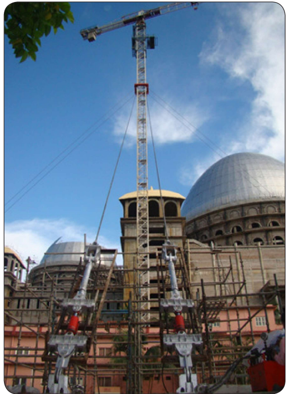
Tower Crane Anchoring System
