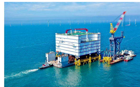
● China Three Gorges Renewable Jiangsu Rudong Converter Station, the first offshore converter station in Asia
