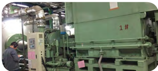
Recovery of waste heat of air compressor operating system and air compressor for heating
