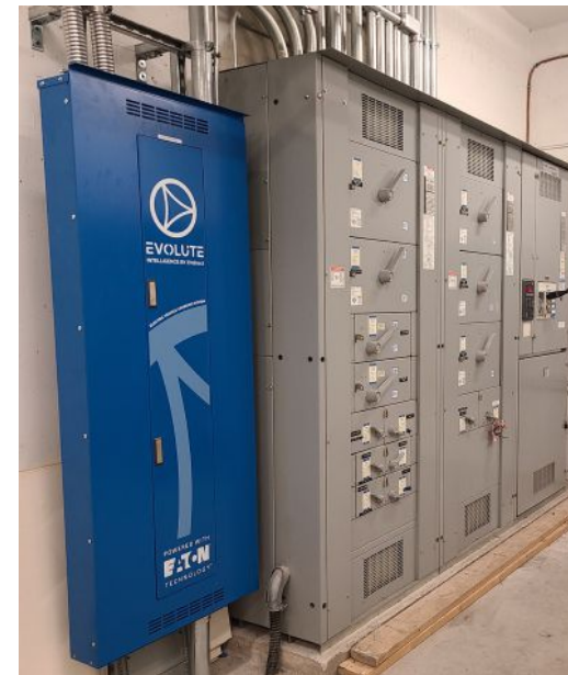
The Evolute is a smart panel system, collaboratively developed between EVdirect and Eaton, to achieve dynamic load management for electric vehicle charging.
