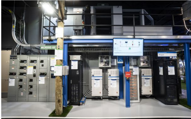
At Eaton's Experience Center in Pittsburgh, a full-scale demonstration and testing facility, you can get a hands-on look at how microgrids support resilience. The controlled environment has a fully functioning building microgrid that interconnects with multiple onsite sources.
